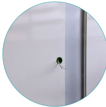
Uncovered installation panel and elektroinstallation
