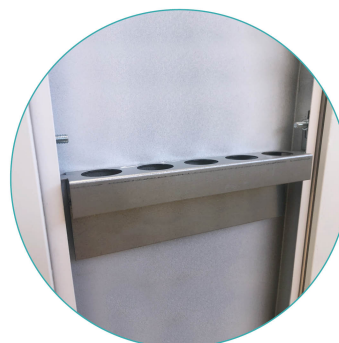
Uncovered installation panel
